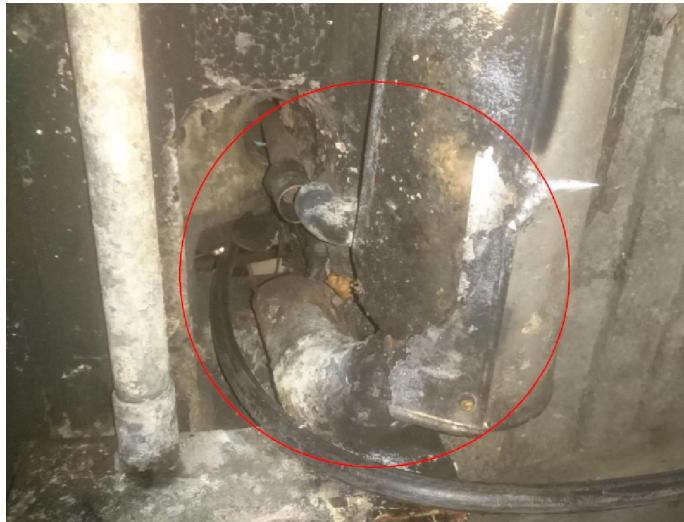
Pic1 Acetylene Pipe
